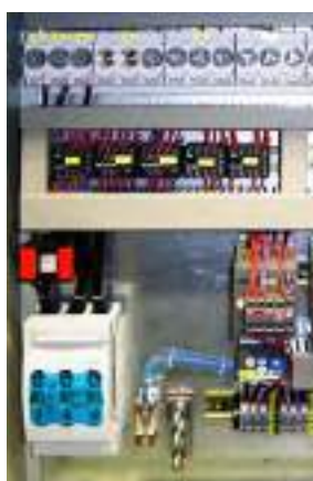
▲ Current converter in switch cabinet
