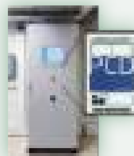
Potential use in primary switch cabinet
