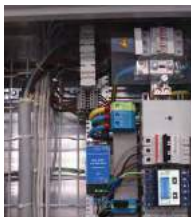
▲ Built-in current converter directly in the cable duct
