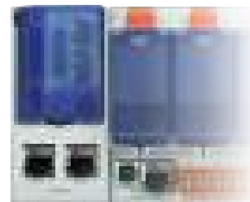
Ethernet 2 (2 port switch)
